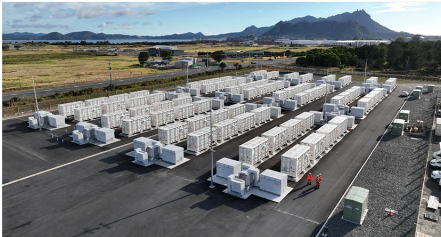
Meridian's Ruakākā Battery Energy Storage System (BESS) is being officially opened in a ceremony later today.
