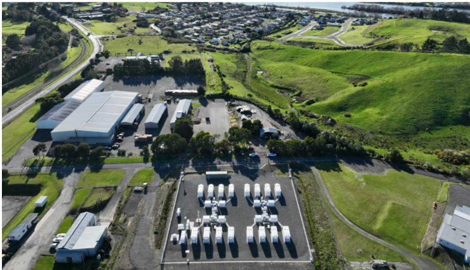
Rotohiko Battery Energy Storage System (BESS) (35 MWh, December, 2023) [ https://infratec.co.nz ]
